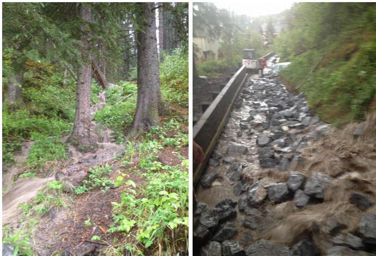
Figure 5-1. Water flowing along the eastern Y Creek diversion wall during the June 2013 event, shown looking upstream (left) and east along the wall (right). Images are stills from a video provided by the Town of Canmore, dated June 19, 2013 at 10:20 am.
