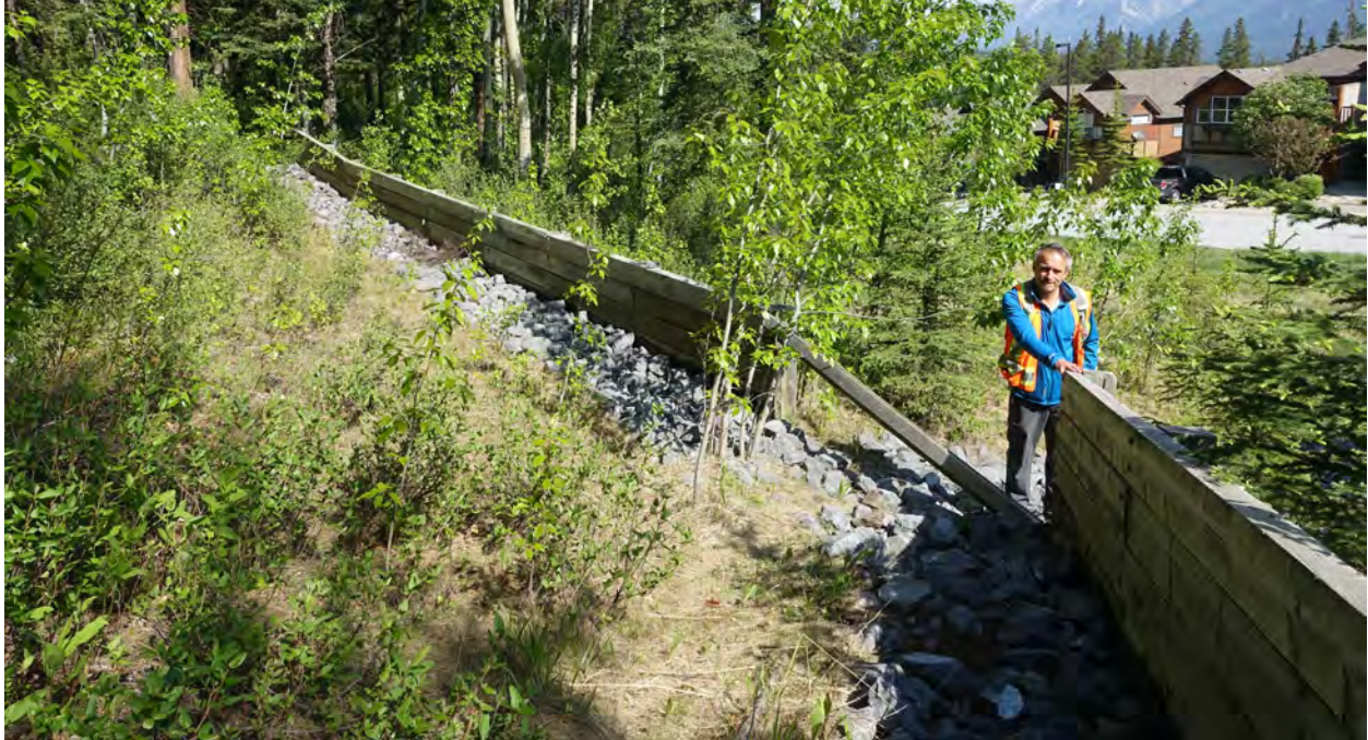
Figure 2-9. Two wooden walls on the western side of the Z Creek fan. The walls are aligned in a V shape, to funnel water into a riprap-lined ditch (Figure 2-10). BGC photo, June 7, 2018.
