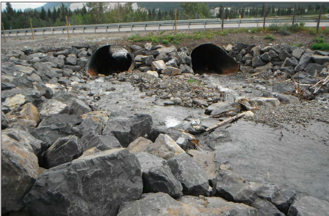
Photo 7130: Looking downstream at the inlet of the upstream pair of Highway 1 culverts.
