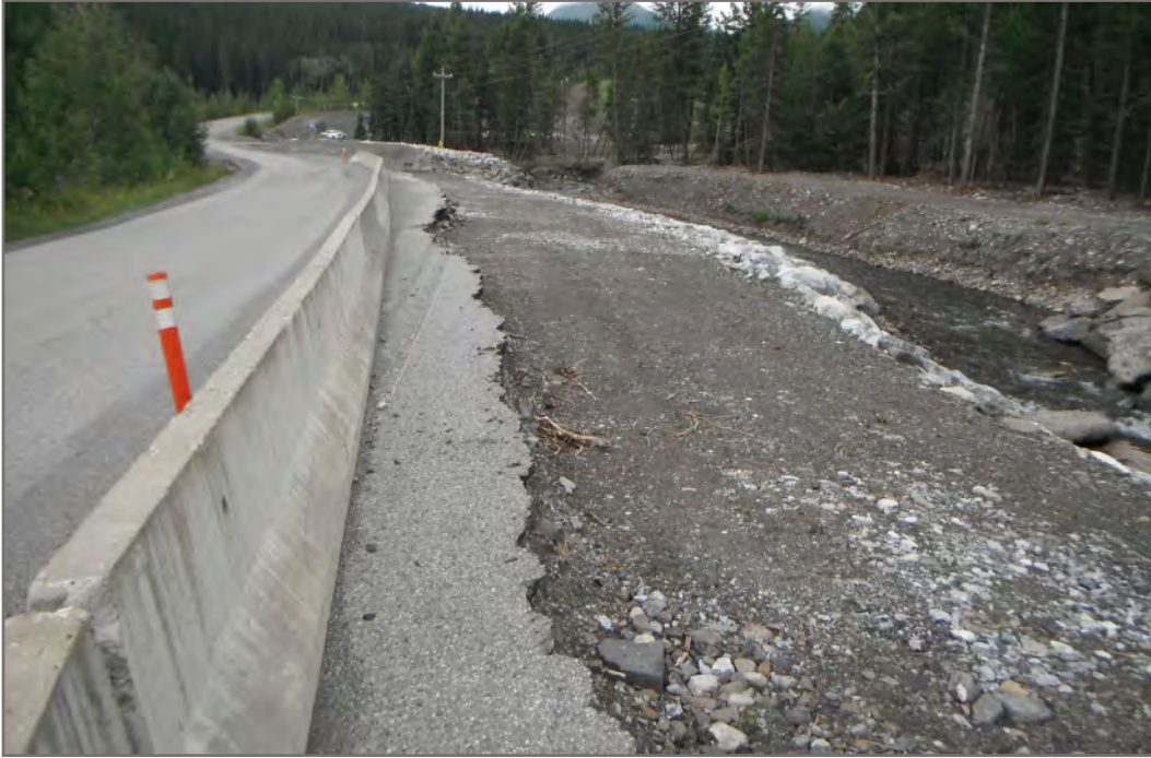
Photo 7137: Damage to George Biggy Senior Road.
