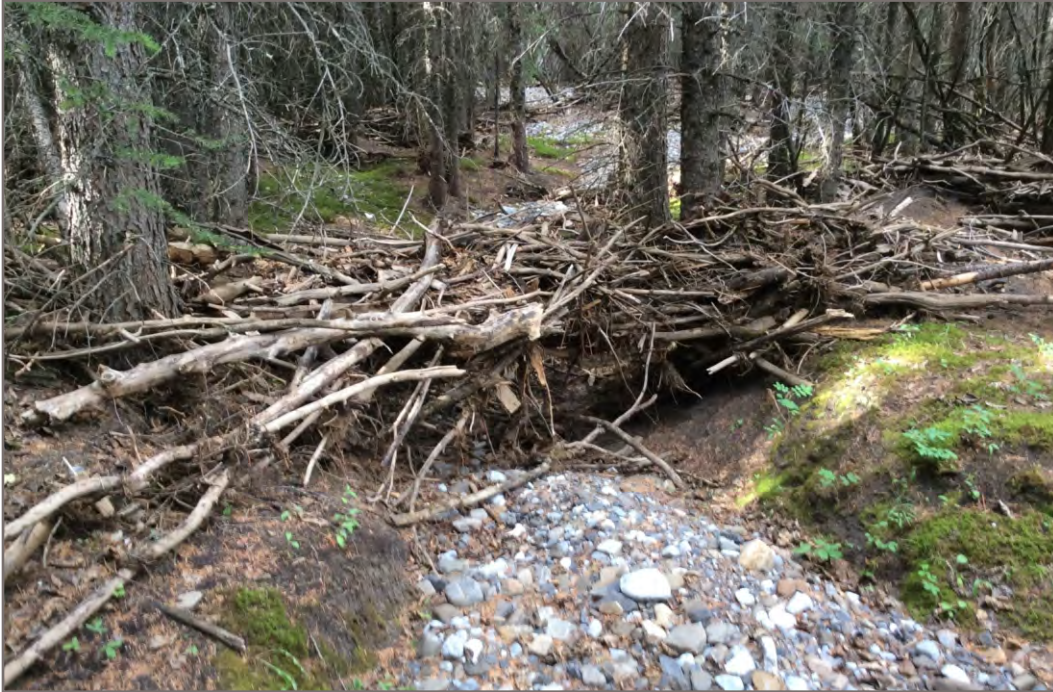
Photo 36(1): Gravel from 2013 event on floor of old channel and log jam showing minimum water level, looking north.
