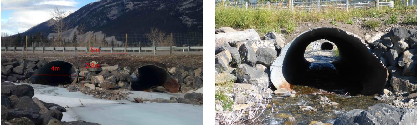
FIGURE 15: HIGHWAY 1 CULVERTS IN MARCH 2015 (LEFT), CULVERT AT THE RAMP IN AUGUST 2015 (RIGHT)
