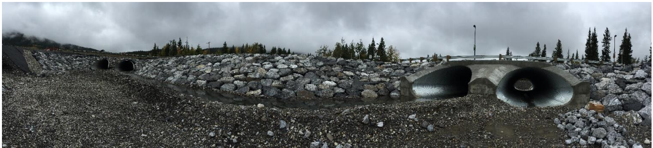
FIGURE 6: STATE OF CHANNEL CONSTRUCTION WORKS IN SEPTEMBER 2016 BETWEEN 2 ND AVENUE AND RIVERS BEND ACCESS
