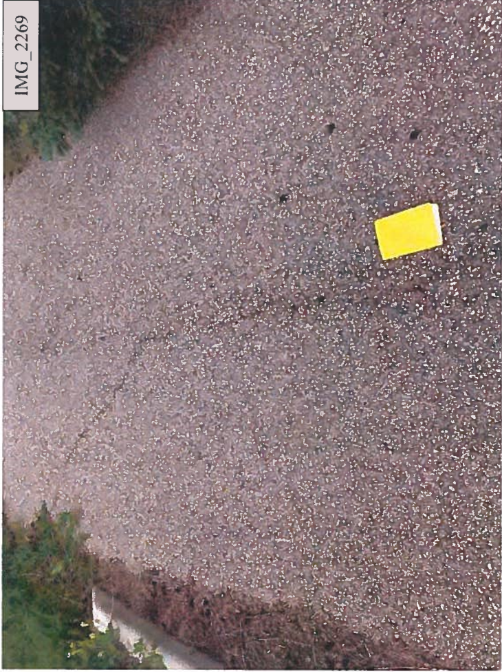
Photograph 7: Slight crack in pathway near feature G903 (waypoints 076 – 083), July 2020
