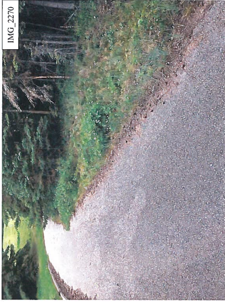
Photograph 8 : Slight crack in pathway near feature G903 (waypoints 076 – 083), July 2020
