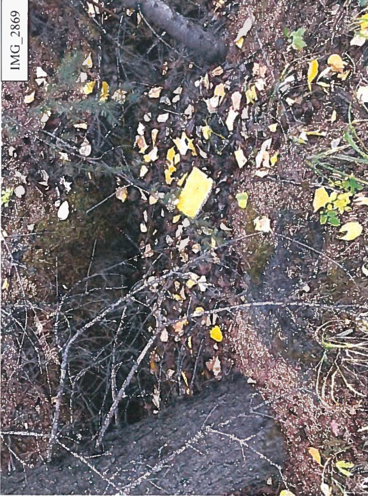
Photograph 47: Possible subsidence area Waypoint 150, September 2020
