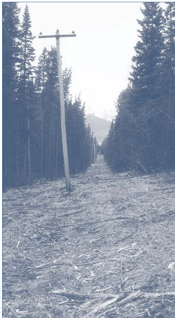
PHOTO: ATCO ELECTRIC
