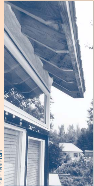
▲ Open eaves, vents not screened. (6 pts)
