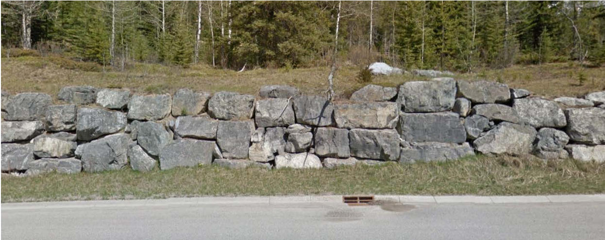
Figure EDCG HLC 9.4: Stone Retaining Wall on Silvertip Road, Canmore AB
