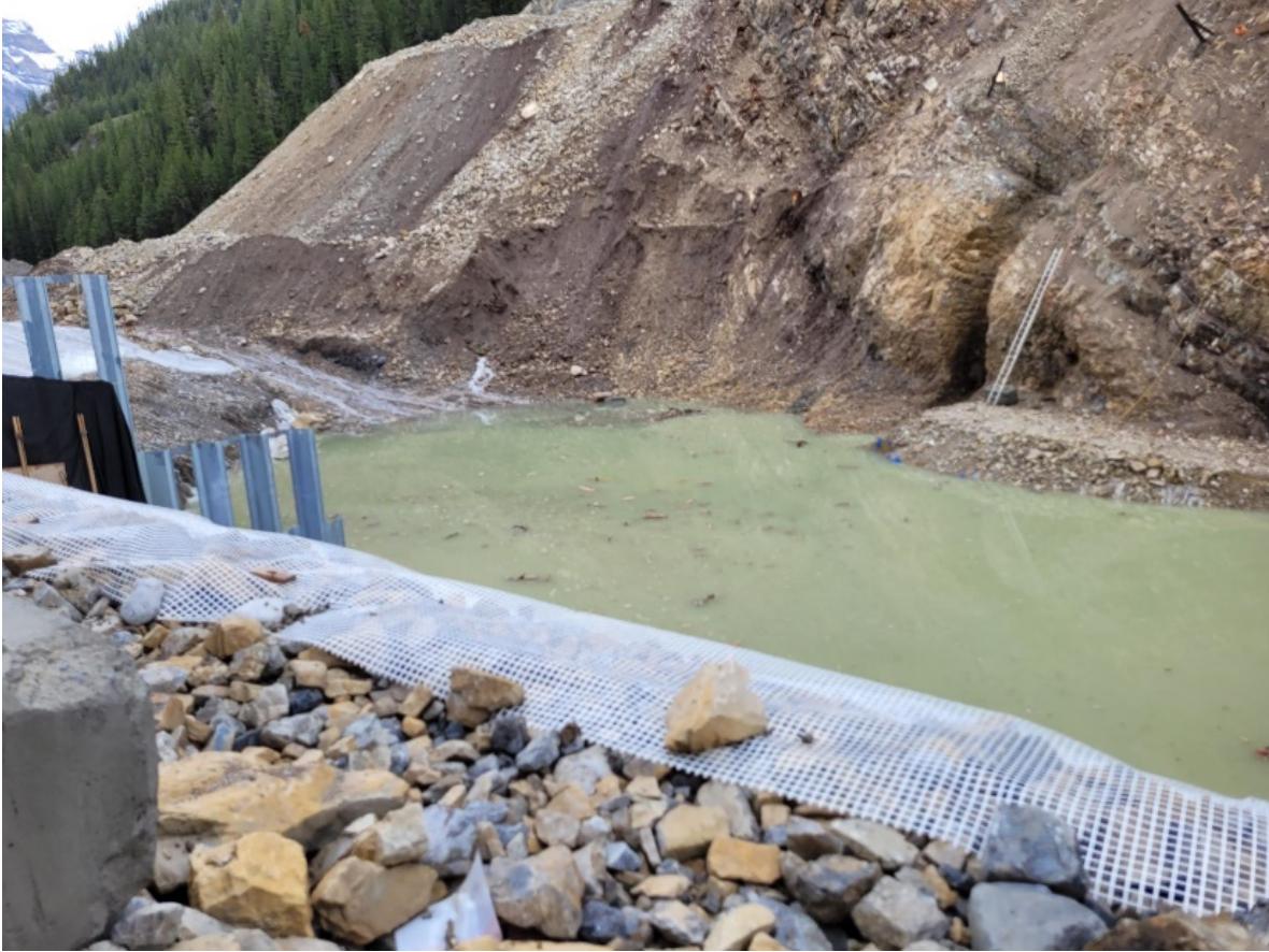
Figure 5: Water filled construction site
