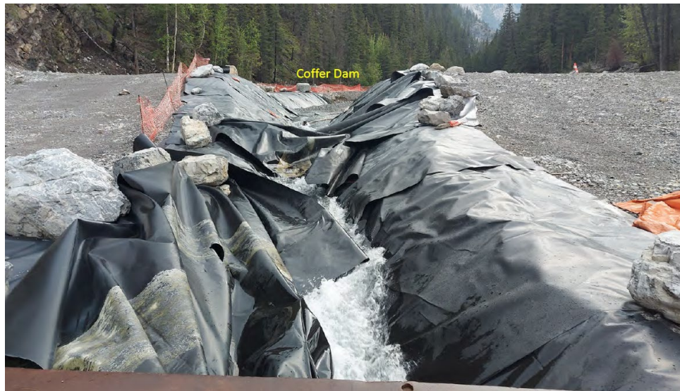
Figure 4: Damaged diversion liner
