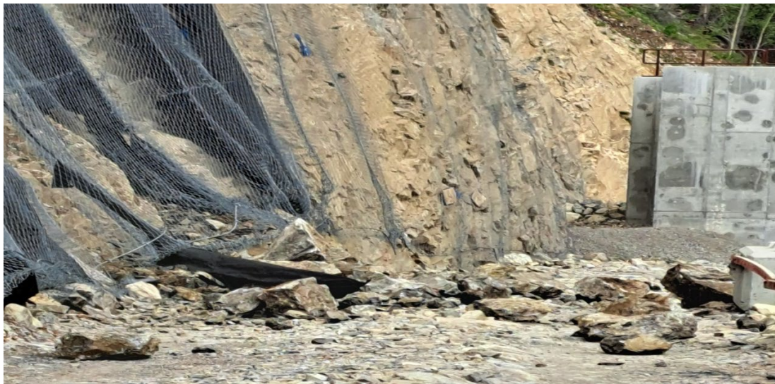
Figure 6: Rockfall on access road
