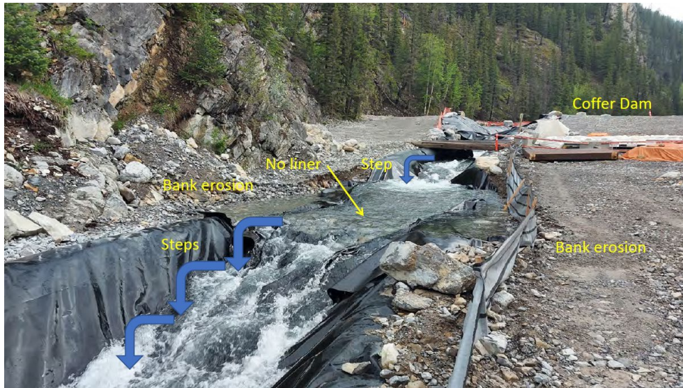
Figure 3: Damaged diversion liner
