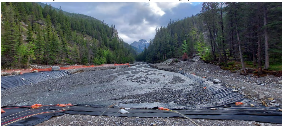
Figure 2: Debris-filled coffer dam
