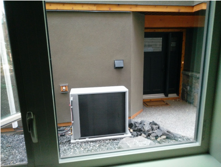
Photograph of air conditioner from adjacent bedroom in South Canmore.
