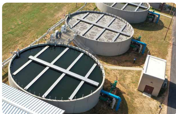
Three AquaNereda® reactors show compact design, typically 50% of a conventional plant.
