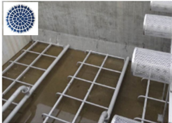
Figure 6: MBBR reactor basin showing internal components, sieves for media retention and MBBR media with dimensions approximately 25 mm diameter x 4 mm thickness (not to scale) (Courtesy of Veolia)
