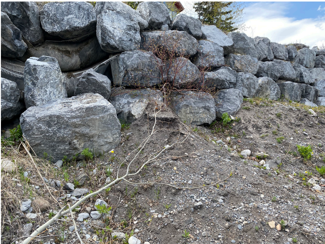
Photograph 2 Base of retaining wall facing at the failed section
