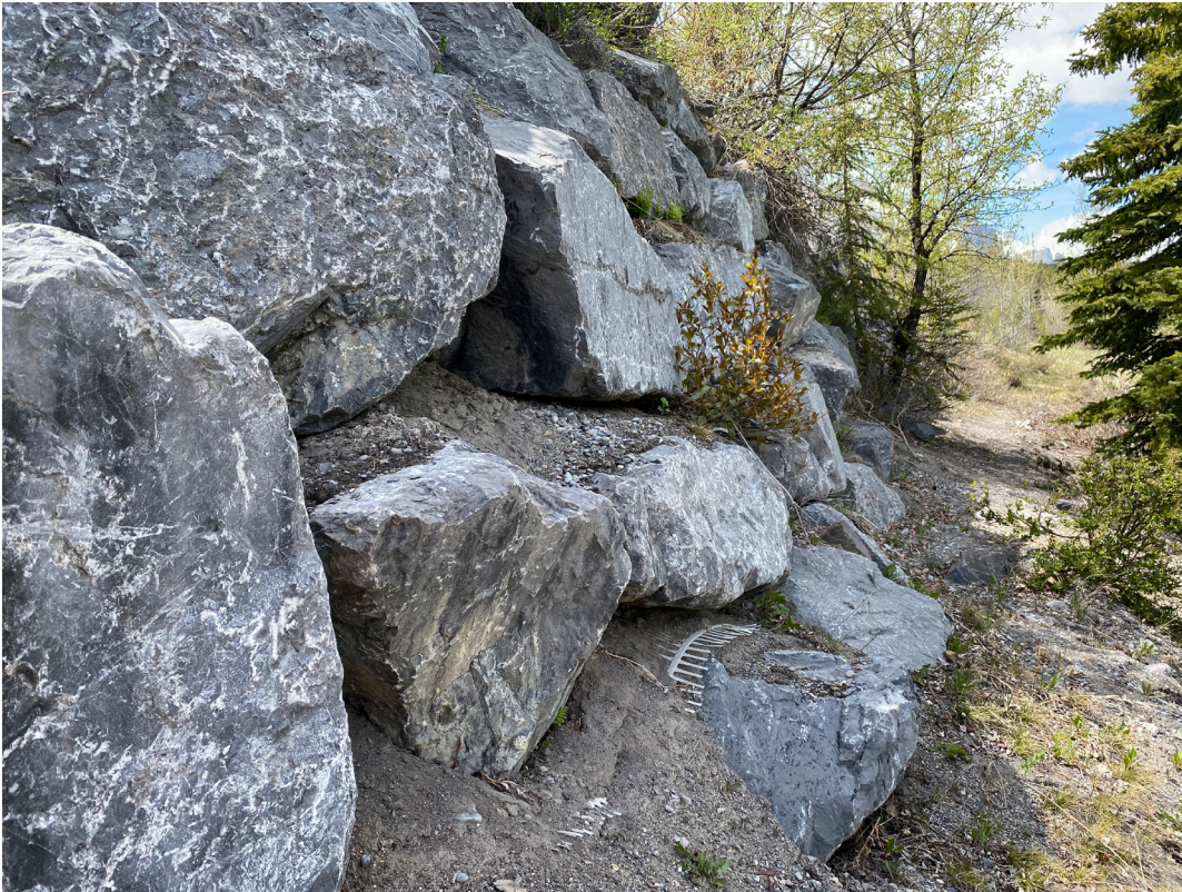
Photograph 3 Washed out fines from the retaining wall
