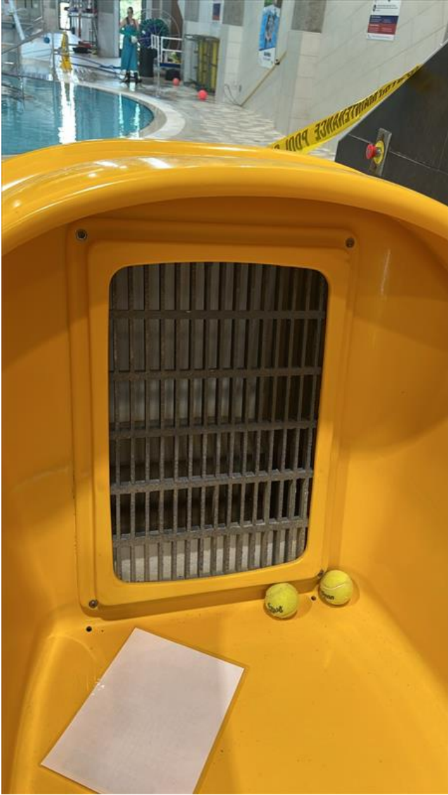
Waterslide Terminal Drain at Base of Slide
