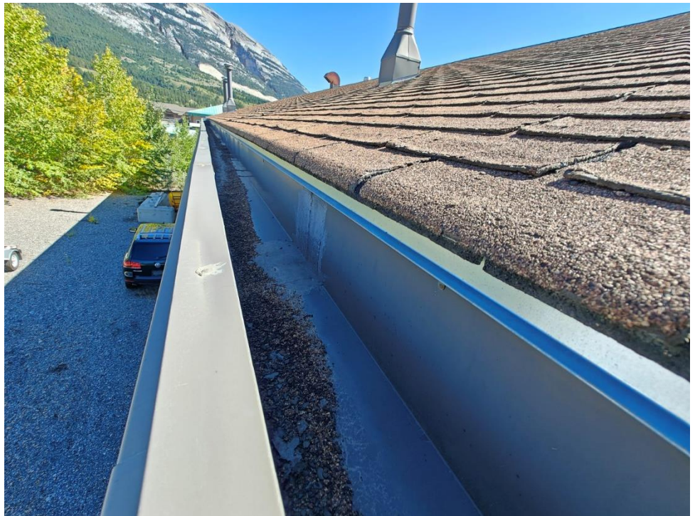
6) Remove all flashings, gutter metal, and drip edge flashing and replace with new.
