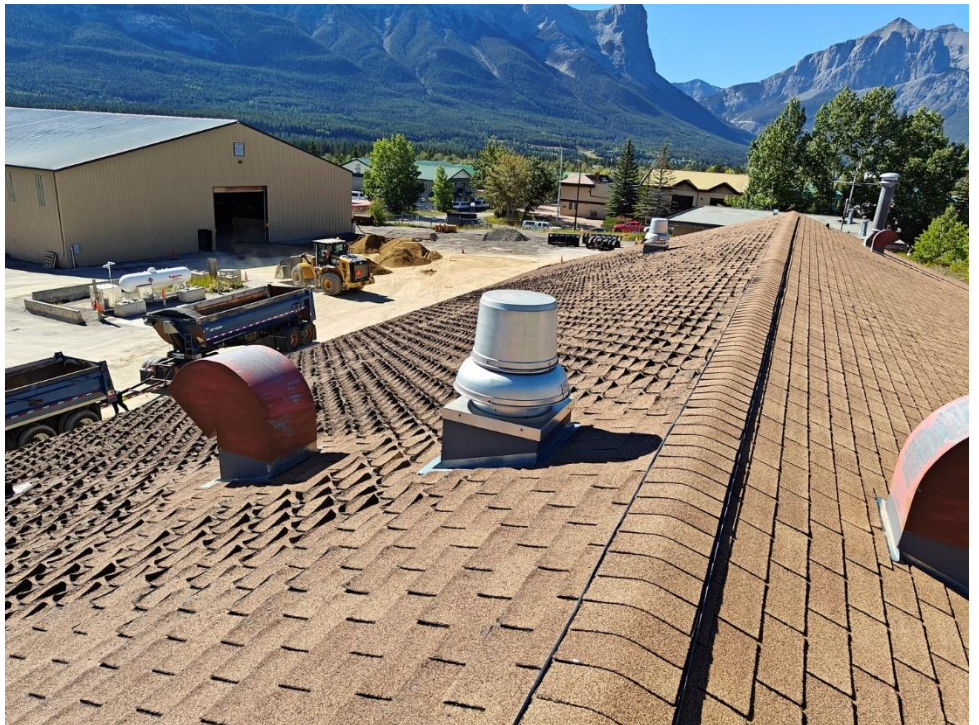
10) Mechanical penetrations to be reflashed with new membrane and metal flashings. Confirm usage with Consultant and Owner.
