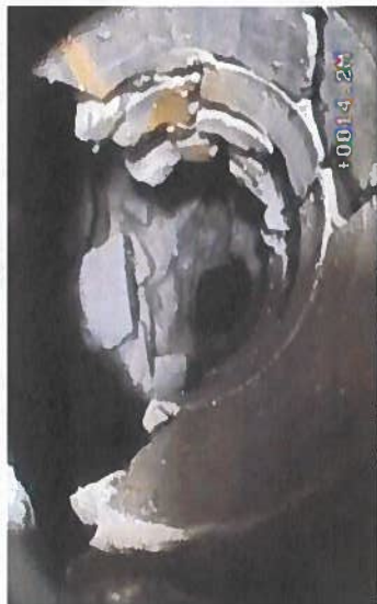
Void at 14.2 to 14.4 m
