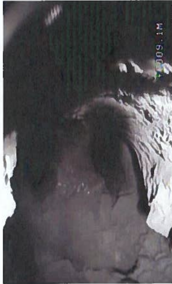
Widening of void at 9.1 m
