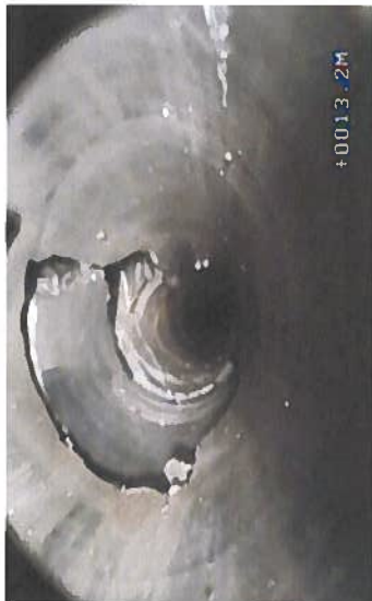
Void at 13.4 to 13.7 m
