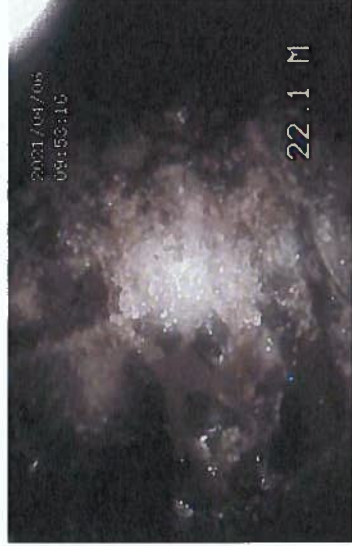
Rubble noted on the floor
