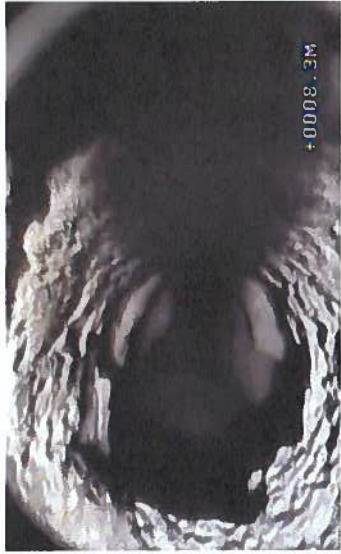
Start of void at 8.4 m
