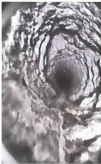
Start of void noted at 27.9 m extending to 29.0 m
