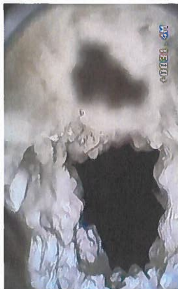
Start of void at 31.7 m
