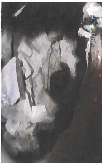
Blocky rubble noted at 14.4 m
