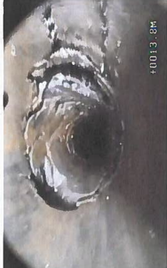
Void at 13.8 to 14.0 m
