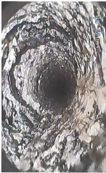
Fractures noted at 29.6 m
