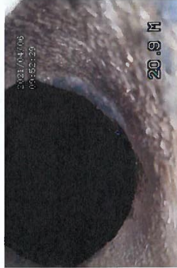
Start of void at 21.1 m
