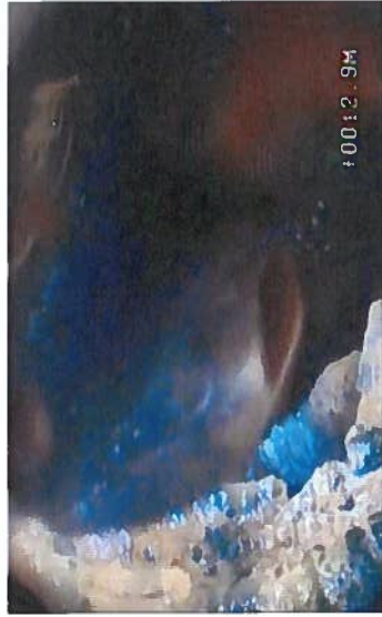
Side view of the void at 12.9 m
