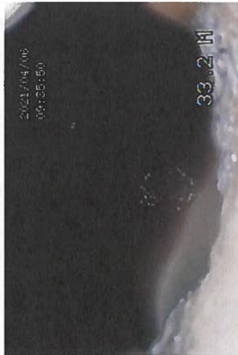
Void at 33.2 to 35.8 m
