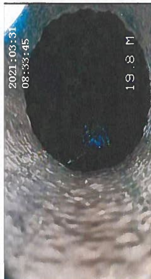
Start of void at 19.8 m
