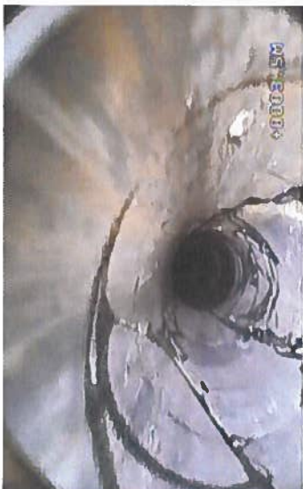
Vertical cracking noted at 3.4 m
