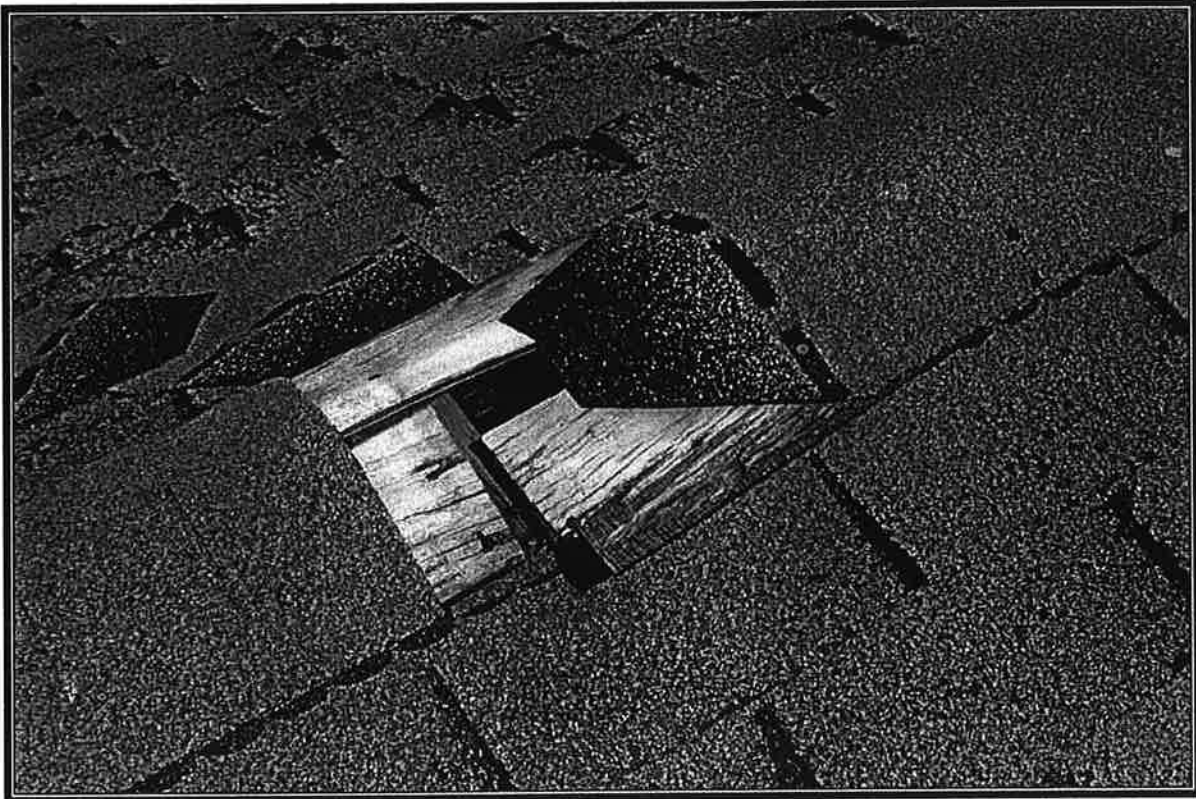
Photograph # 4: Missing ridge cap
