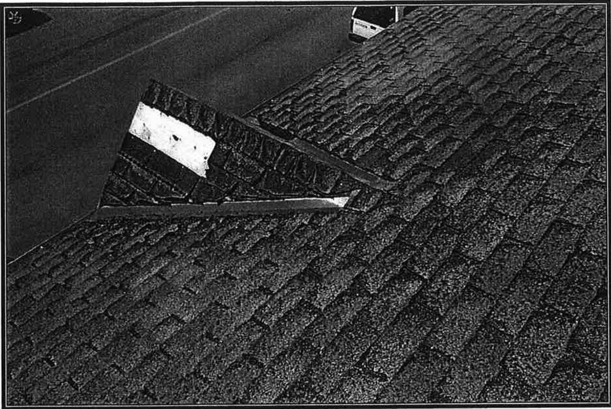
Photograph # 3: Missing shingles
