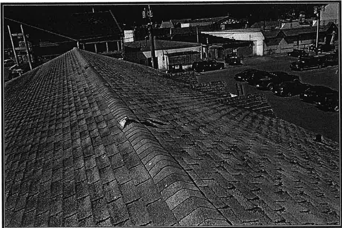
Photograph # 2: Shingles no longer provide an effective water shed
